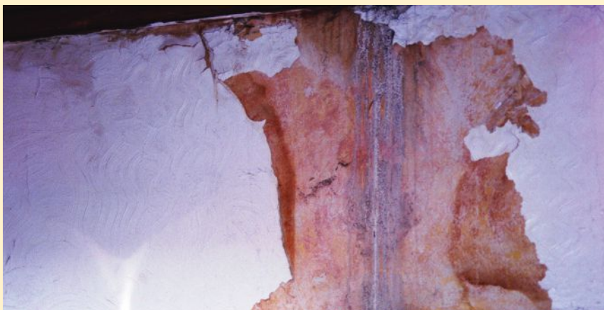
An example of some of the worst damage to the St. Andrew's, Beacon sanctuary walls.
